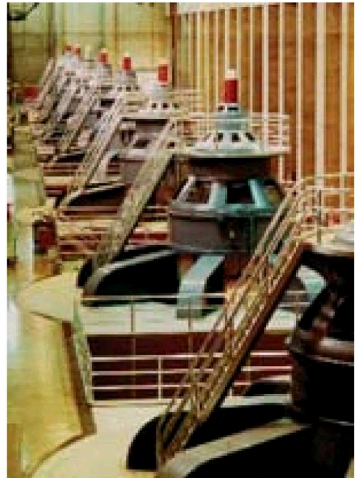
A series of hydel generators.
